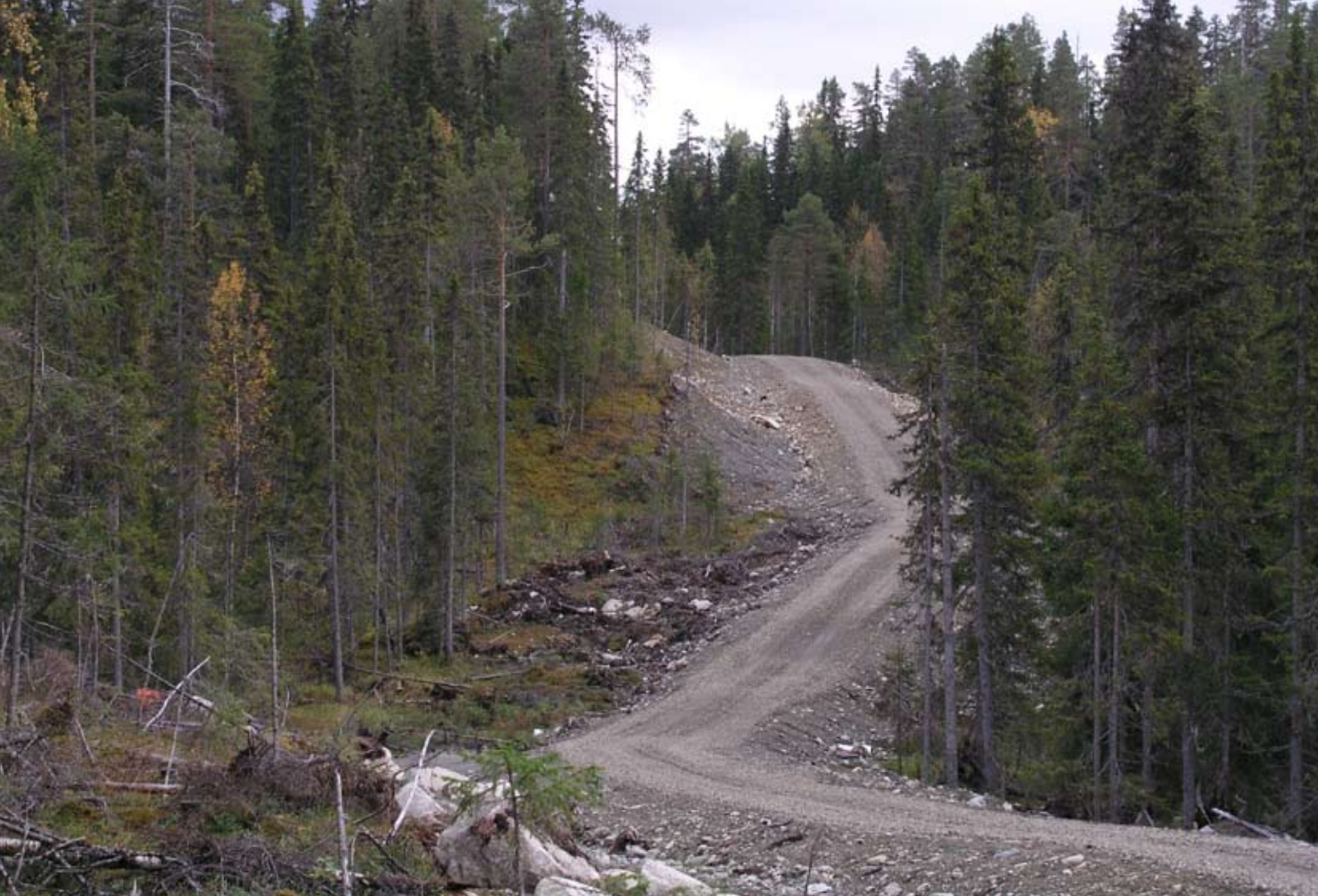
A service road built by SCA through a forest on Bräntkullarna that, determined by the Swedish Forest Agency, is a WKH. SCA had planned to clear cut the valuable forest. Photo: Olli Manninen
