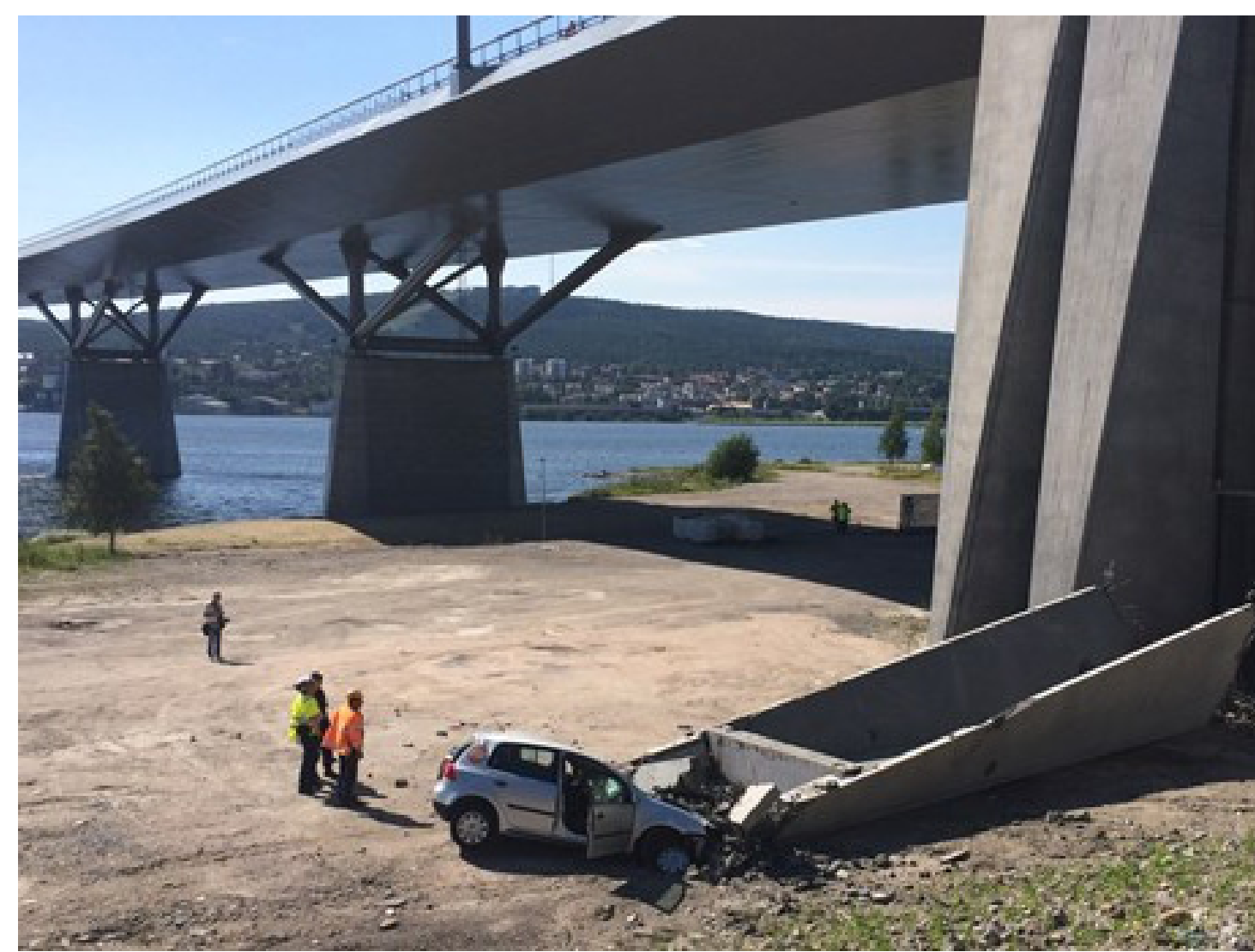
Fig. 1. A 30-tonne block of concrete suddenly fell out of the newly built bridge in Sundsvall in August 2015. http://www.svt.se/nyheter/regionalt/vasternorrland/br-opelare-rasade-over-bil
